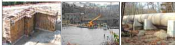
Brewer Professional: Brewer, ME | Amoskeag Hydro: Manchester, NH | Jackman Penstock Replacement: Hillsborough, NH
